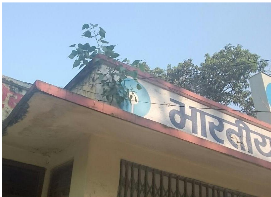
Figure2. Young plant of Ficus religiosa on wall of the building of State Bank of India (Shopping Center Branch) on the Banaras Hindu University main campus
